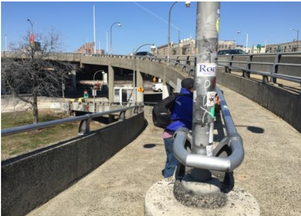
Narrow widths and constricted turns at existing access ramp
