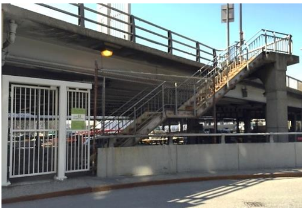
Existing condition at NY-North: W. 179 th Street and Cabrini Boulevard: lack of crosswalk and entry area with buffer from street, stair access-only
