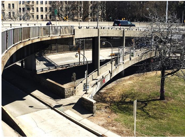
Existing condition at NY-South: W. 178 th Street and Cabrini Boulevard: absence of entry area and street buffer; ramp access to bridge is narrow with constricted turns
